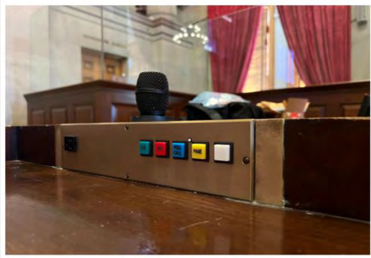
Tennessee House: New face plates, switches, and electronics are designed to compliment existing elements of the desk furniture and previous console insert.
