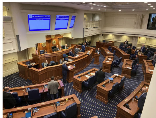
Alabama Senate — Existing P.A. (public address) speakers to the upper left and right of rostrum while new, taller aimable speaker arrays are positioned lower to better broadcast sound to those listening anywhere on the chamber floor.
